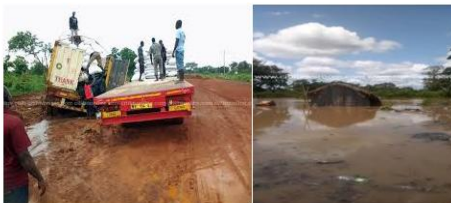
Photo 7: Road infrastructure damaged by floods in Wulensi, Nanumba South District
