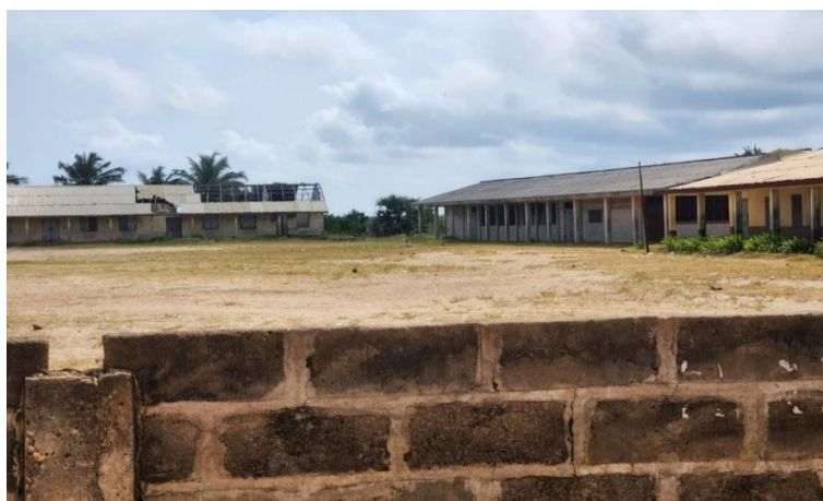
Photo 6: School buildings affected by rainstorms at Woe-Afedome
