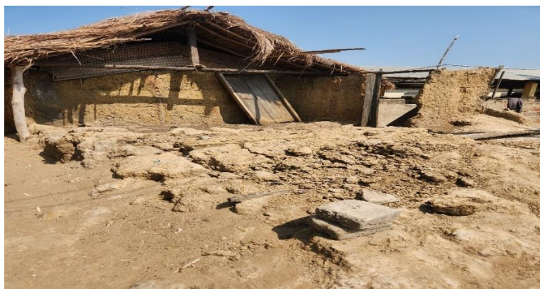
Photo 5: Mudhouse damaged by floods at Bleamezado
