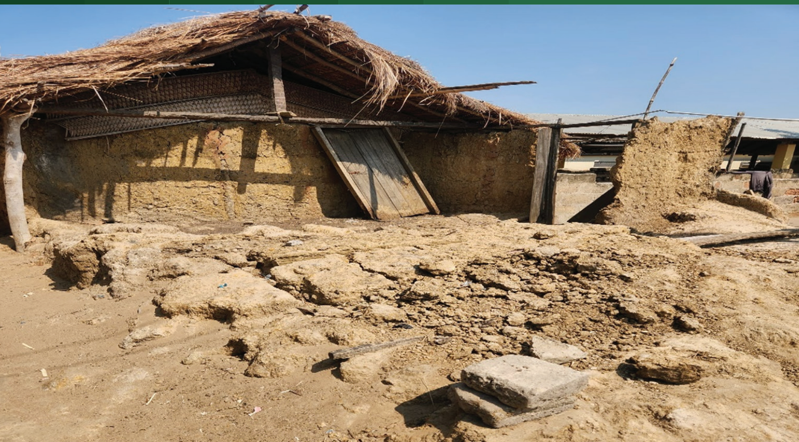
Plate 1: Mudhouse damaged by floods at Bleamezado Credit: Desmond Adjason, 2024
