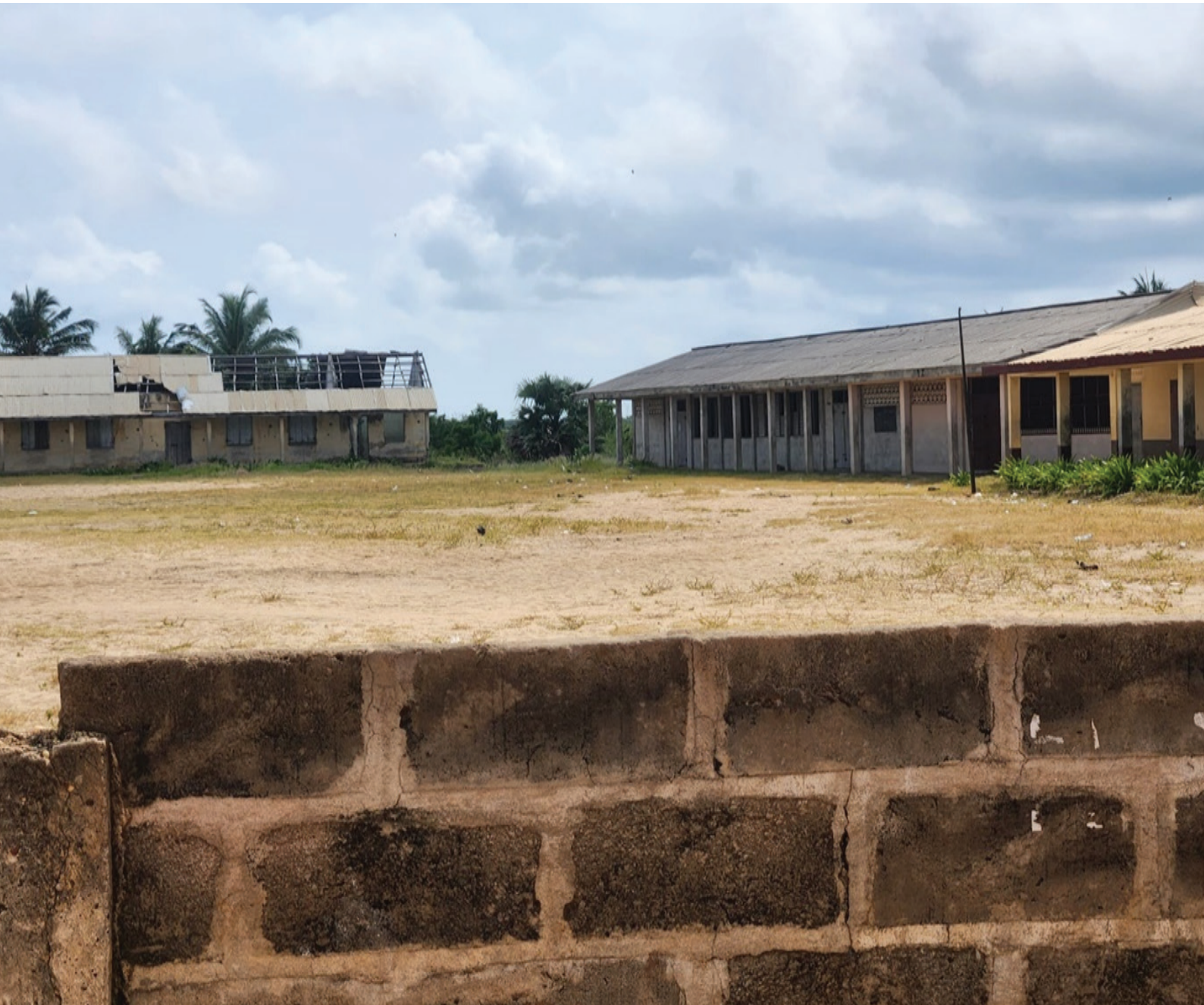
Plate 7: Classrooms in Anloga left roofless and abandoned due to severe rainstorms in the district. Credit: Desmond Adjason, 2024
