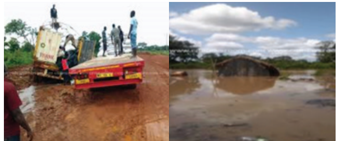
Plate 5: Road Infrastructure damaged by floods in Wulensi, Nanumba South District Credit: Antwi-Agyei and team, 2024
